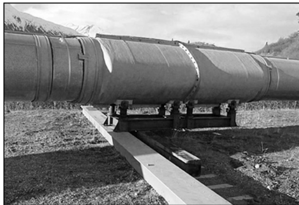
Figure 12. Pipe shoe at Denali Fault crossing perched at edge of grade beam support following fault displacement.
