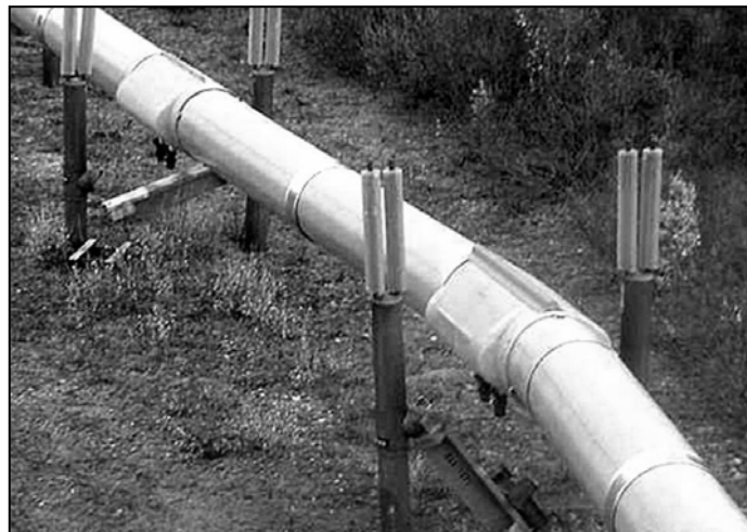
Figure 7. Loss of two adjacent supports on above-ground pipeline near Denali Fault. The possible loss of two adjacent supports was a fundamental design assumption.
