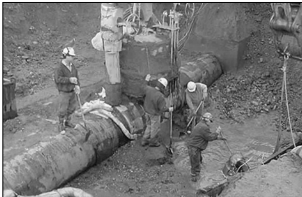
Figure 9. Pipeline and remote gate valve excavated at liquefaction zone. There was no evidence of damage or movements were well within tolerable limits.
