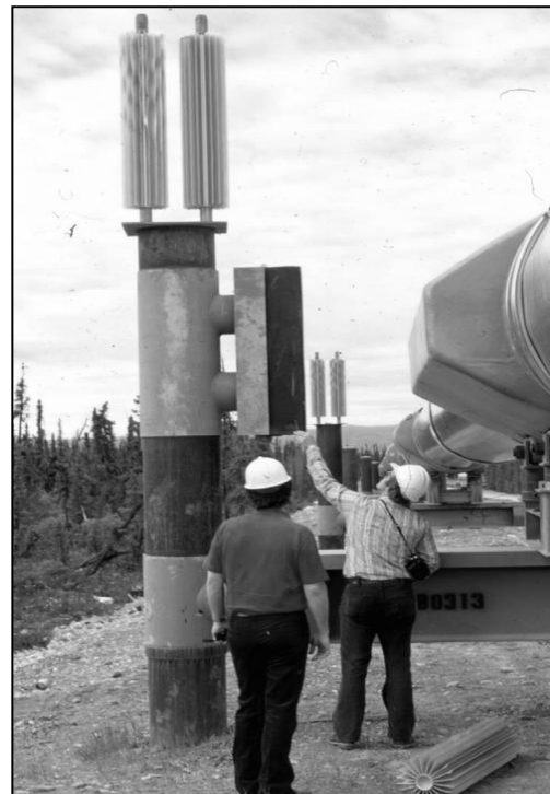
Figure 5. Bumper restraint to control lateral seismic movement.
