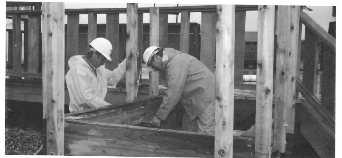
Norcon Laborers Mike Linden and Dennis Kendall worked through the cold autumn rains to construct the disabled access ramp at the Yukon River visitor information pavilion.
